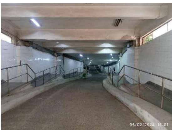
Platinum Jubilee Underpass between 203 BT Road and 202 BT Road of ISI, Kolkata. Fund sanctioned for this as well as construction completed during his directorship.
